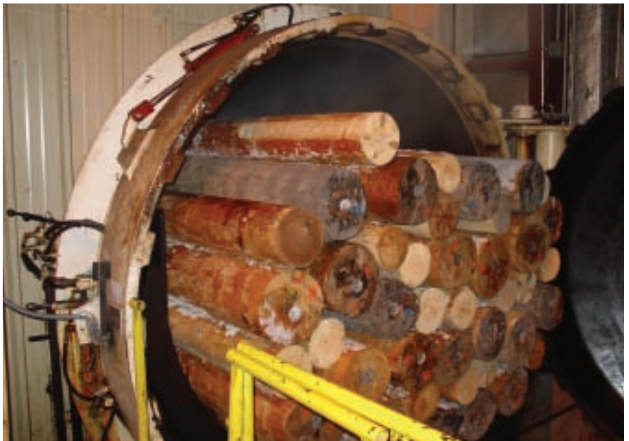
Red Pine poles that were peeled, seasoned, and framed at the Barron plant now enter New Brighton's treatment cylinder.
