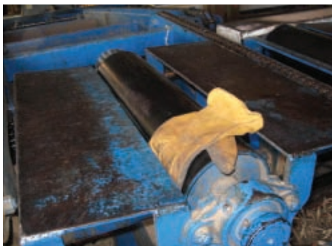
Pinch point on a roller system
