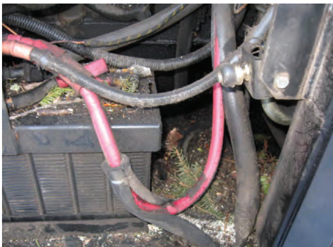
This picture shows where daily housekeeping would improve fire and personnel safety as well as being able to uncover maintenance needs.
