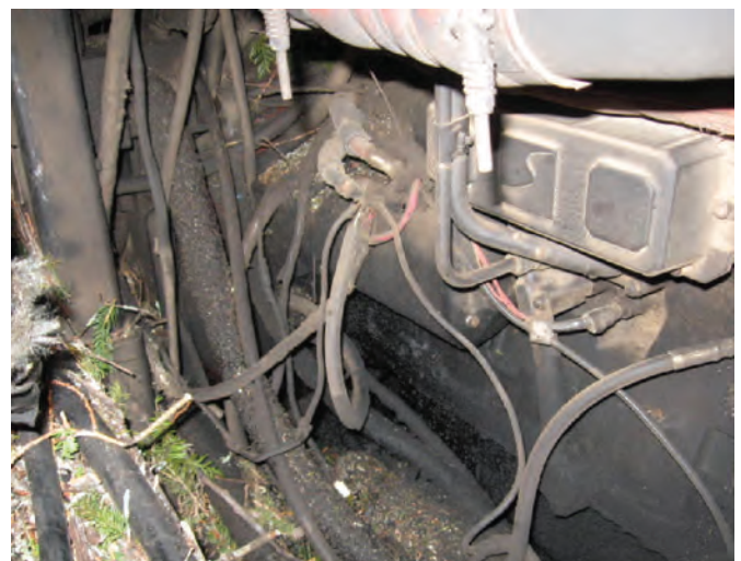
This picture demonstrates the need for improved daily housekeeping and a routine power wash.
