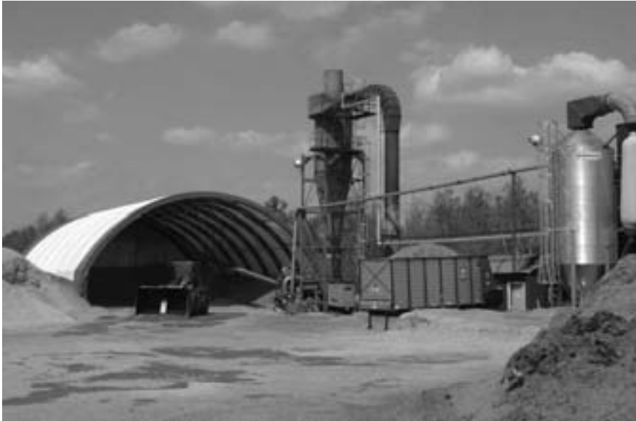
The drier behind Woodline dries chips and residue to be used for biomass. The material is stored under the white dome until it's ready to be shipped.
