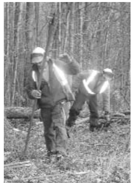
Darren Hughes, foreman, and John Duffey, ground laborer, clearing trees near lines south of Grand Rapids.
