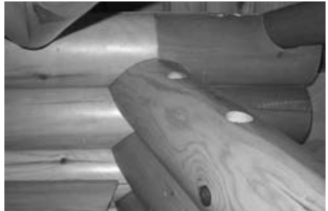
A view of the pre-drilled bolt holes that help make Northwoods Log Home so stable.
