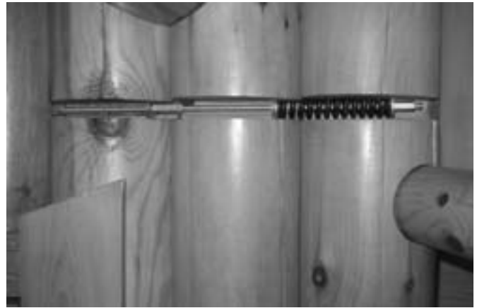
A compression spring is part of the 14-course column that involves independent fasteners and thru-bolting.
